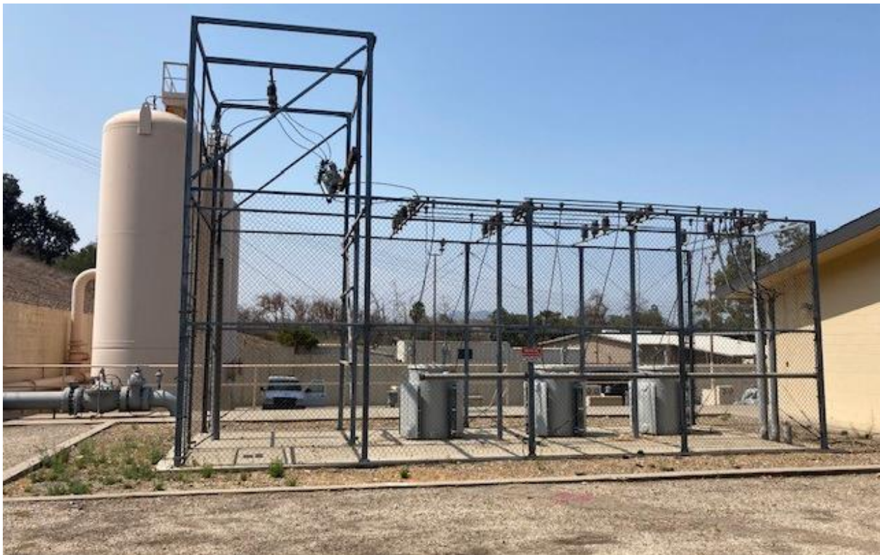
Figure 6 View of Electric Substation Equipment, View South
