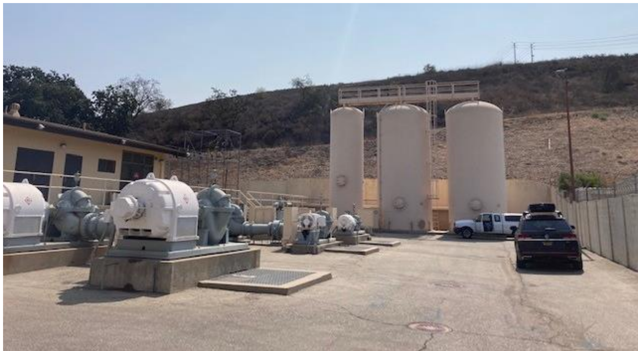
Figure 2 View of Pump Tanks and Surge Tanks, View Northeast
