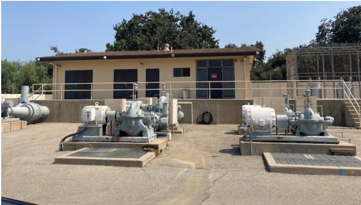
Figure 4 View of Control Building South Elevation with Pump Trains, View North
